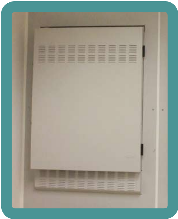
To comply with the ADA protrusion requirements and maintain appropriate enclosure depth, the enclosures were recessed into the wall.
